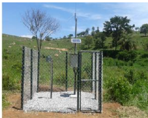
Figure 17: Pluviographic station and data logger
