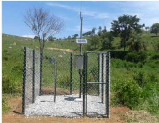
Figure 17: Pluviographic station and data logger
