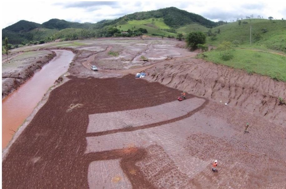
Figure 43: Preparation of the soil utilizing manual and semi-mechanized methods of scarification of the substrate, seeding and fertilization being executed near Paracatu de Baixo
